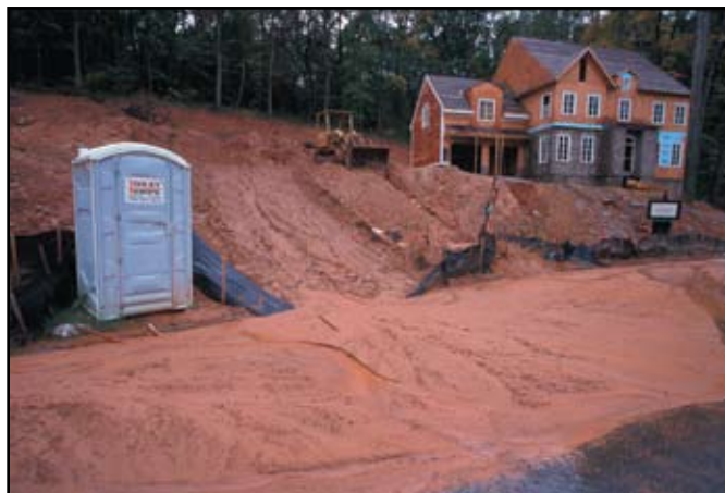
Sedimentation, a pervasive form of aquatic habitat degradation throughout much of North America, here results from poorly regulated construction in the Nancy Creek system, a Chattahoochee River tributary in metropolitan Atlanta (1997).
